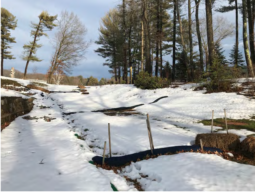
Fig 9: Slope above the manhole at Gundalow Landing/east side of the bay. Viewing east. (03-01-21)
