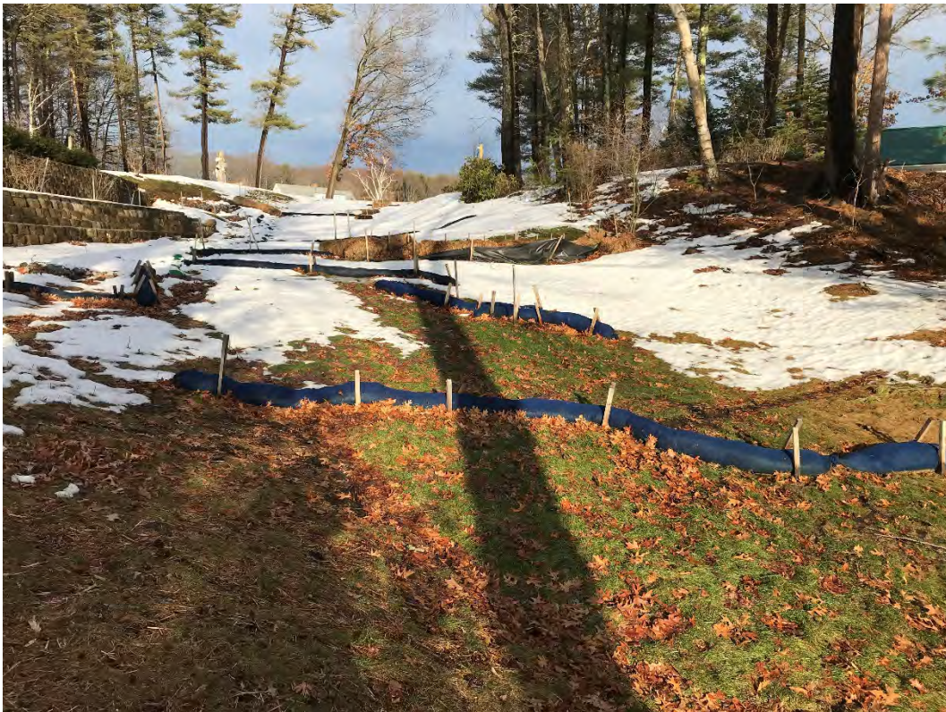
Fig 10: Slope below the manhole at Gundalow Landing/east side of the bay. Viewing east. (03-01-21)
