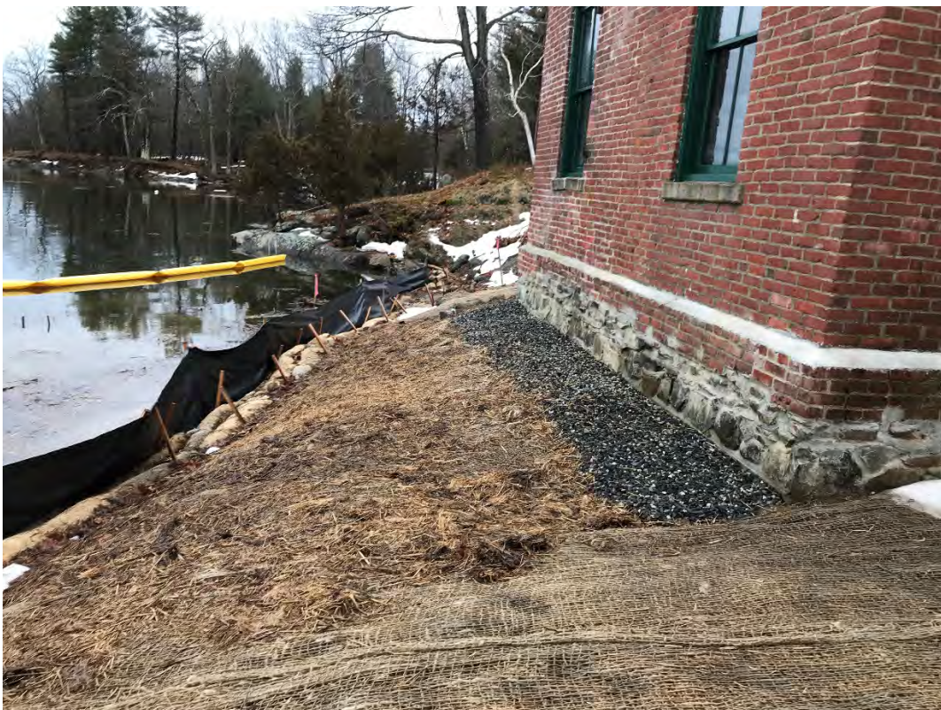
Fig 2: Slope between the cable house and salt marsh restoration at the Eversource property/west side of the bay. Viewing south. (03-01-21)
